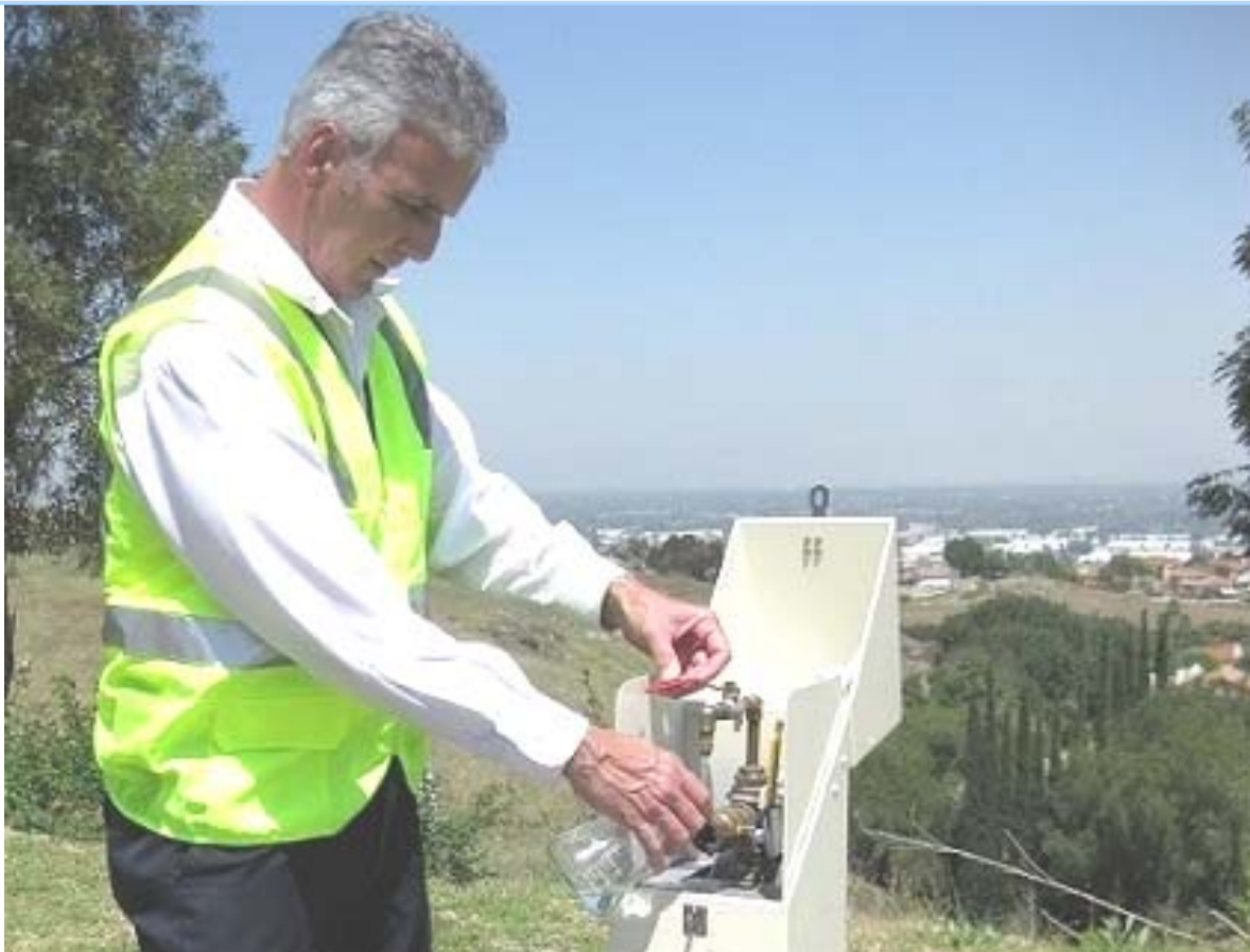
1 of 35 Pomona distribution samples sites. Over 22,000 water quality tests performed in 2014 to meet SWRCB DDW standards.
